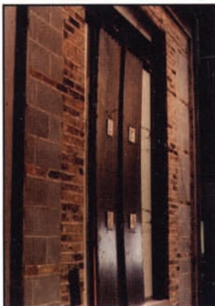
During test, with fire on corridor side – note distortion of door toward flame, due to heat
